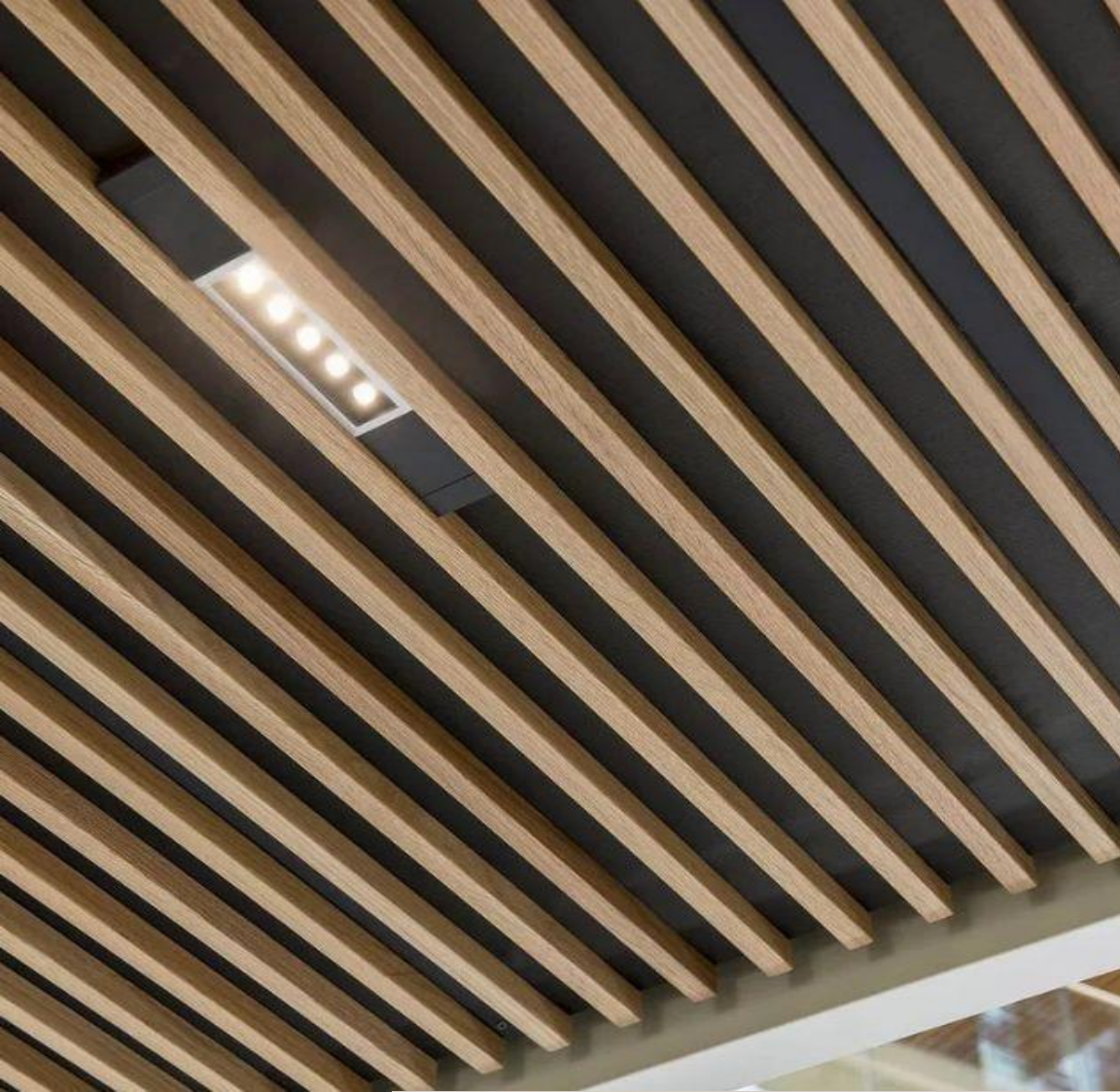
Wooden Suspended Ceiling
